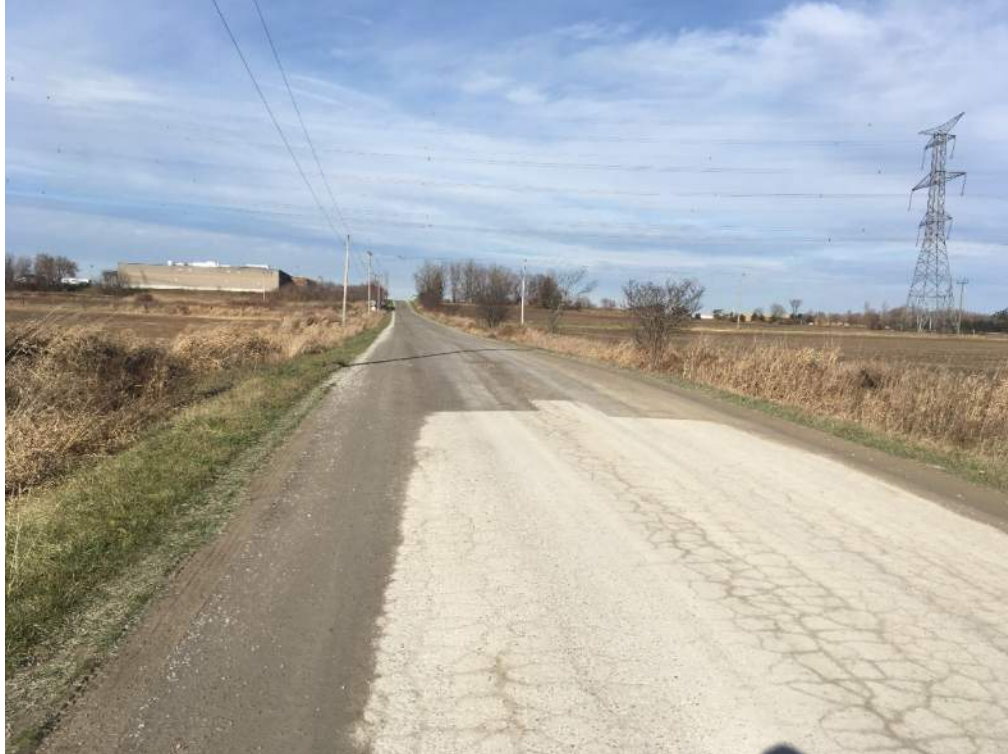
Photo 15: Poor asphalt conditions on north road approach with loose gravel and pavement cracks.
