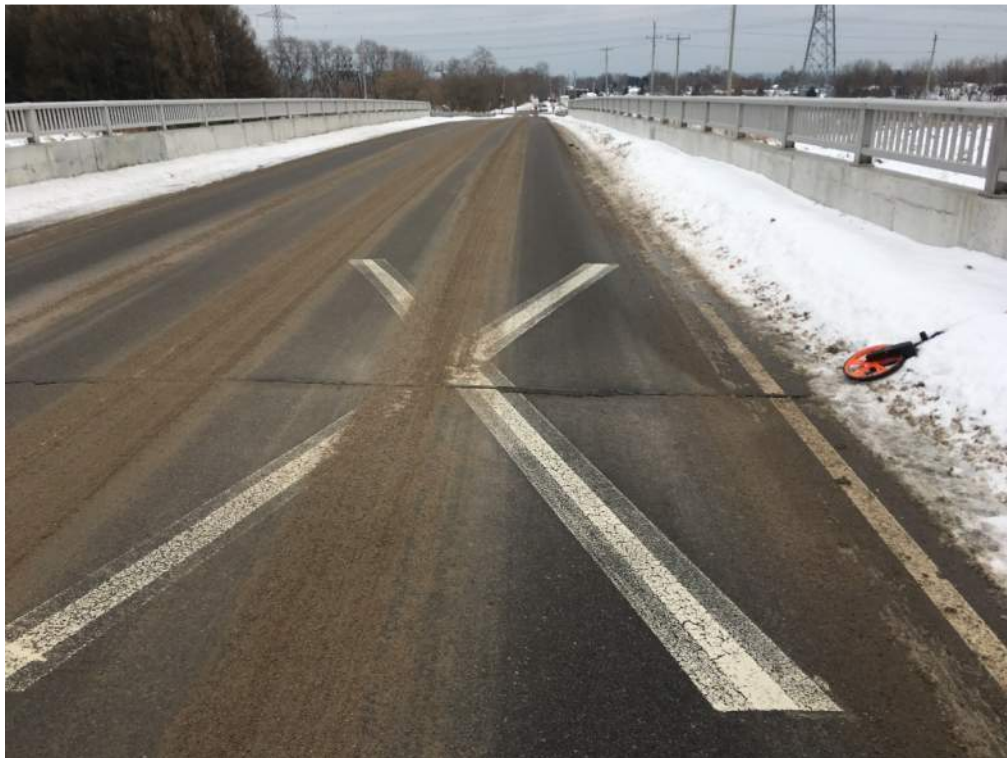
Photo 22: North road approach, "X" pavement marking at 180m from crossing and is faded.
