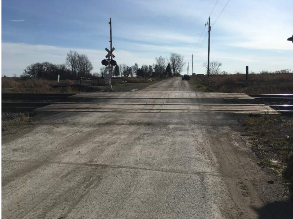
Photo 13: Gradient through crossing, looking south. Uneven transition between north road approach and crossing, with positive gradient through crossing towards south road approach.
