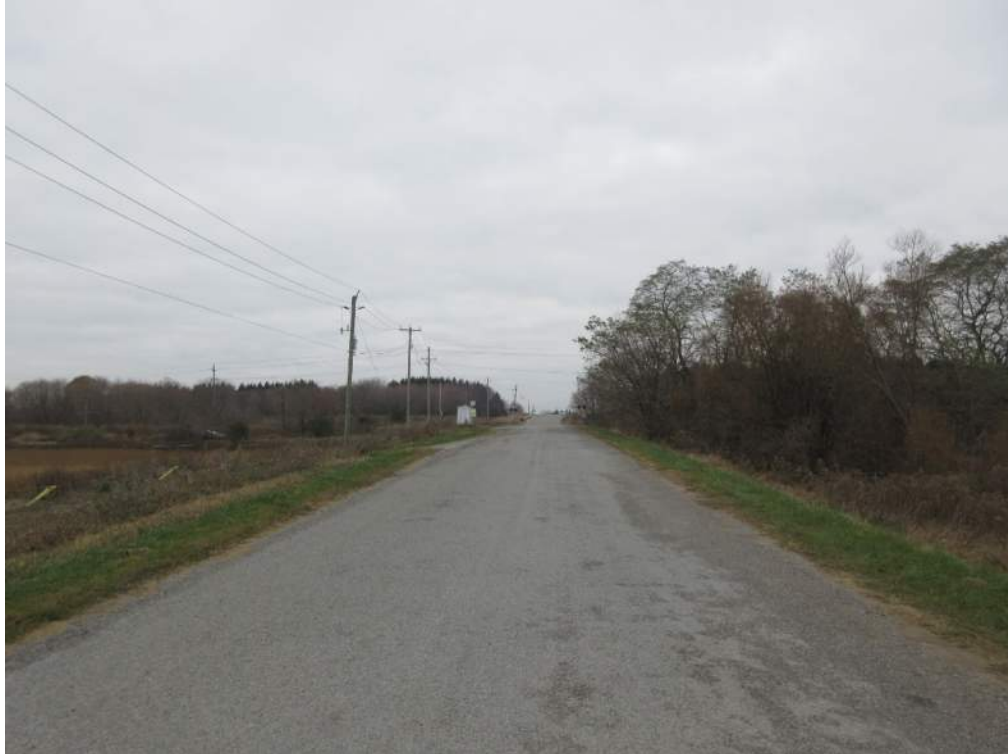
Photo 15: View of crossing at SSD of 110m for road speed of 50km/h on the south road approach. “X” pavement markings are not present.
