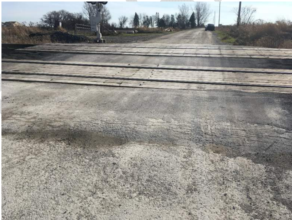
Photo 14: Poor transition from north road approach to crossing surface.
