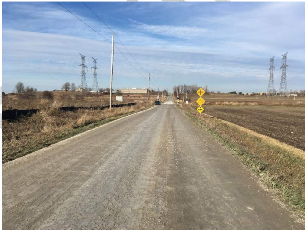
Photo 22: South road approach, crossing at SSD of 110m for road speed of 50km/h. “X” pavement markings are not present.
