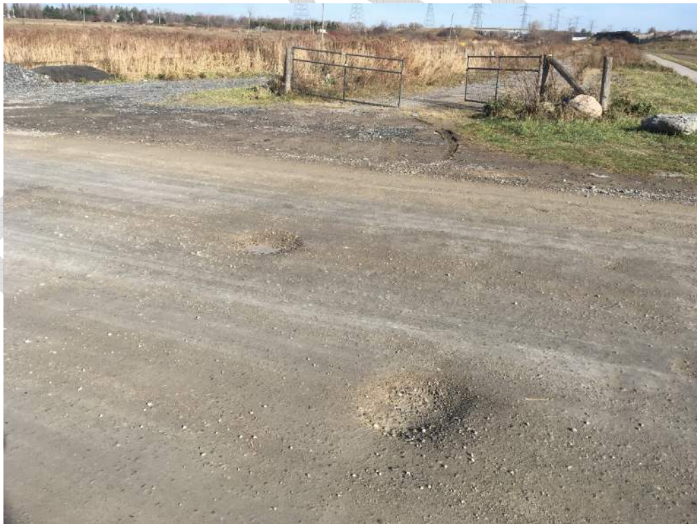
Photo 16: Poor asphalt conditions on south road approach with loose gravel and potholes present.
