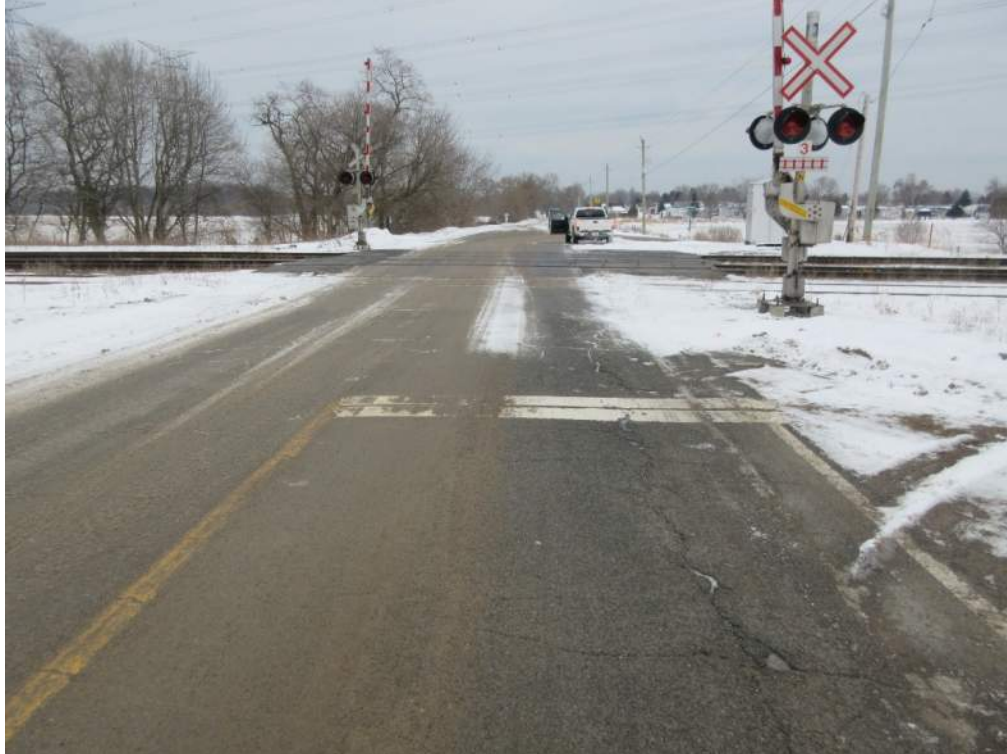
Photo 19: Faded stop bars on the north road approach.
