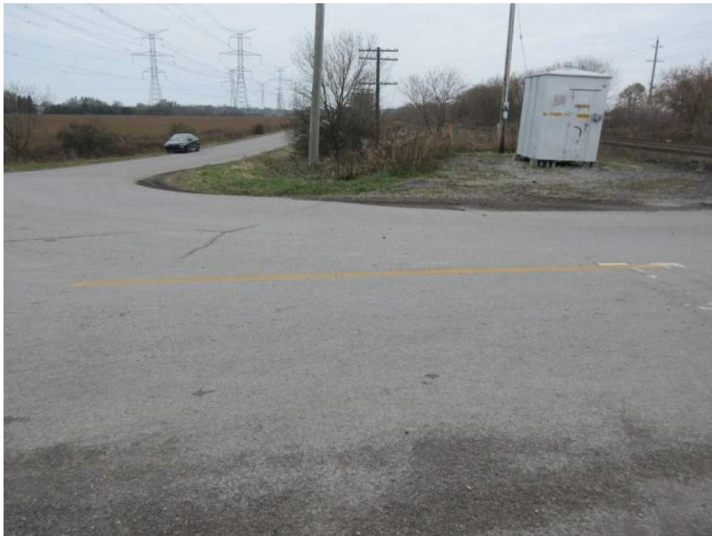
Photo 20: Directional dividing line present and measured to be less than 30m due to close proximity of the Service Road intersection on the south road approach.
