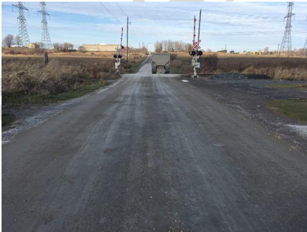
Photo 26: Truck traversing crossing, required to slow down to safely navigate through crossing due to uneven transition and grade changes through crossing. Stop bars are not present on the south road approach.
