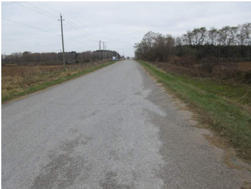
Photo 16: Completely faded “X” pavement marking located beyond 110m on the south road approach.
