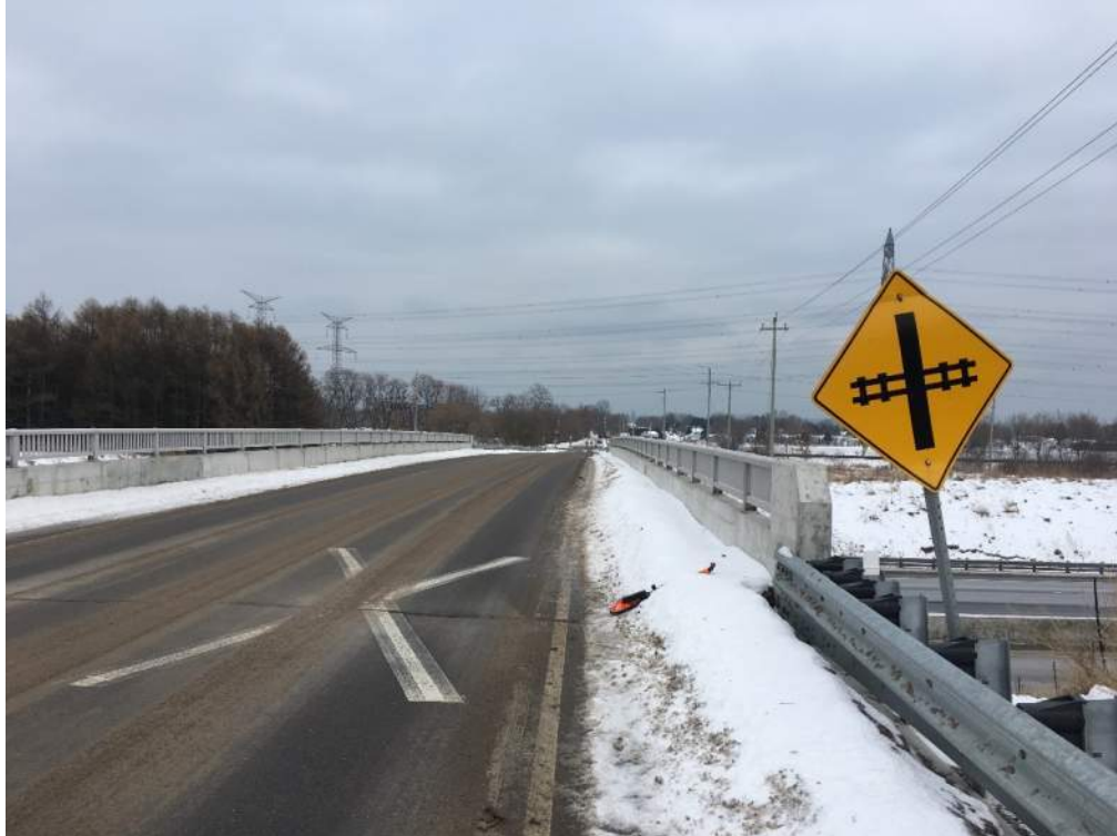
Photo 23: North road approach, WA-18 sign placed within 10m of corresponding “X” pavement marking. Sign is leaning, damaged and does not show correct number of tracks.
