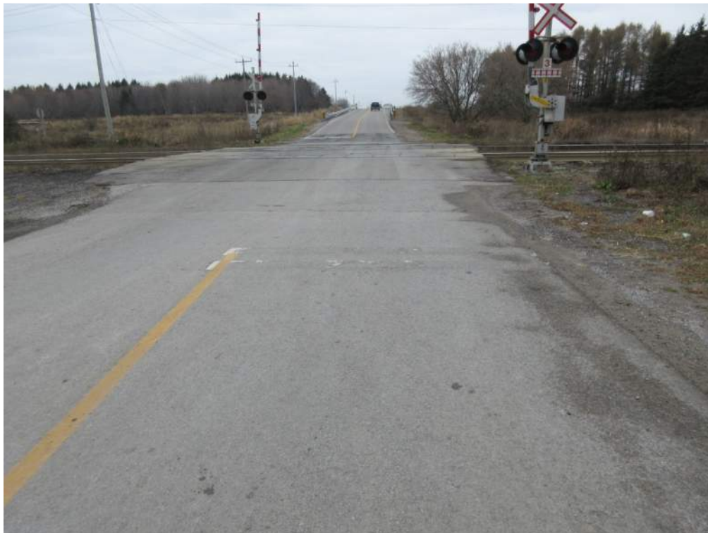
Photo 18: Faded stop bars on the south road approach.
