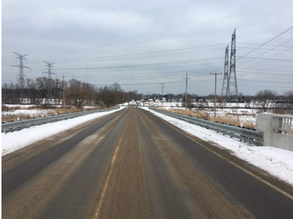
Photo 21: View of crossing at SSD of 110m for road speed of 50km/h on the north road approach.
