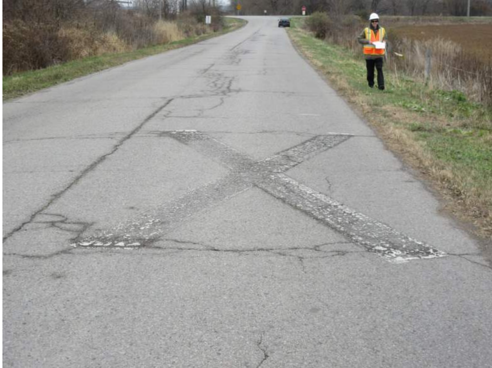
Photo 25: "X" pavement markings on Service Road are heavily faded.
